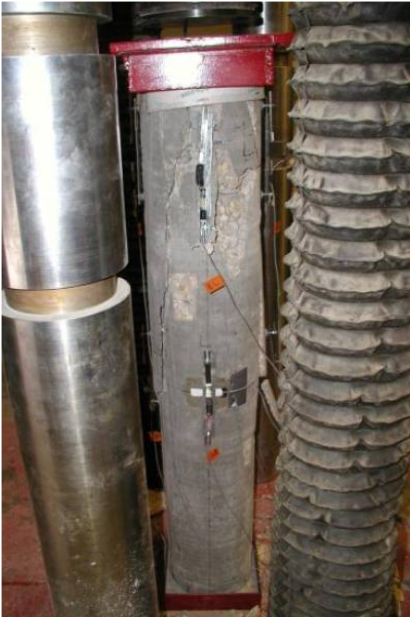
Figure 65: Column FF-FAC after failure.
